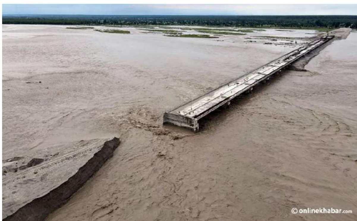
Figure 3: A section of Dam washed away by flood in Mahakali river in an under construction Bridge (Source: Onlinekhabar)
