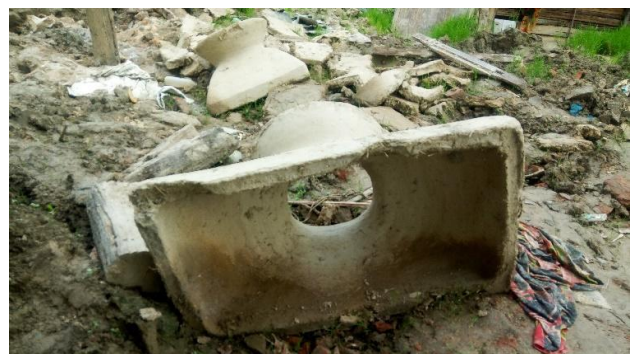
Figure 1: A flood damaged house with its damaged mud-mortar rice container
